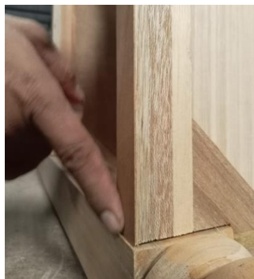
Gambar 4. Sambungan antar komponen tidak rata Figure 4. Uneven joints between components
